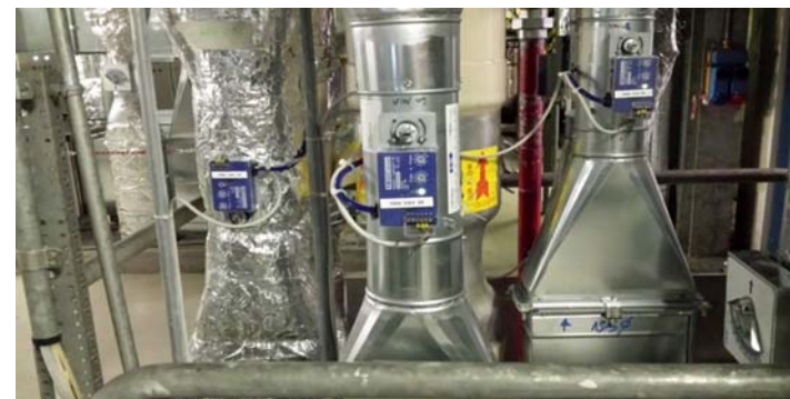
Grade B/C/D rooms' variable air volume regulators
